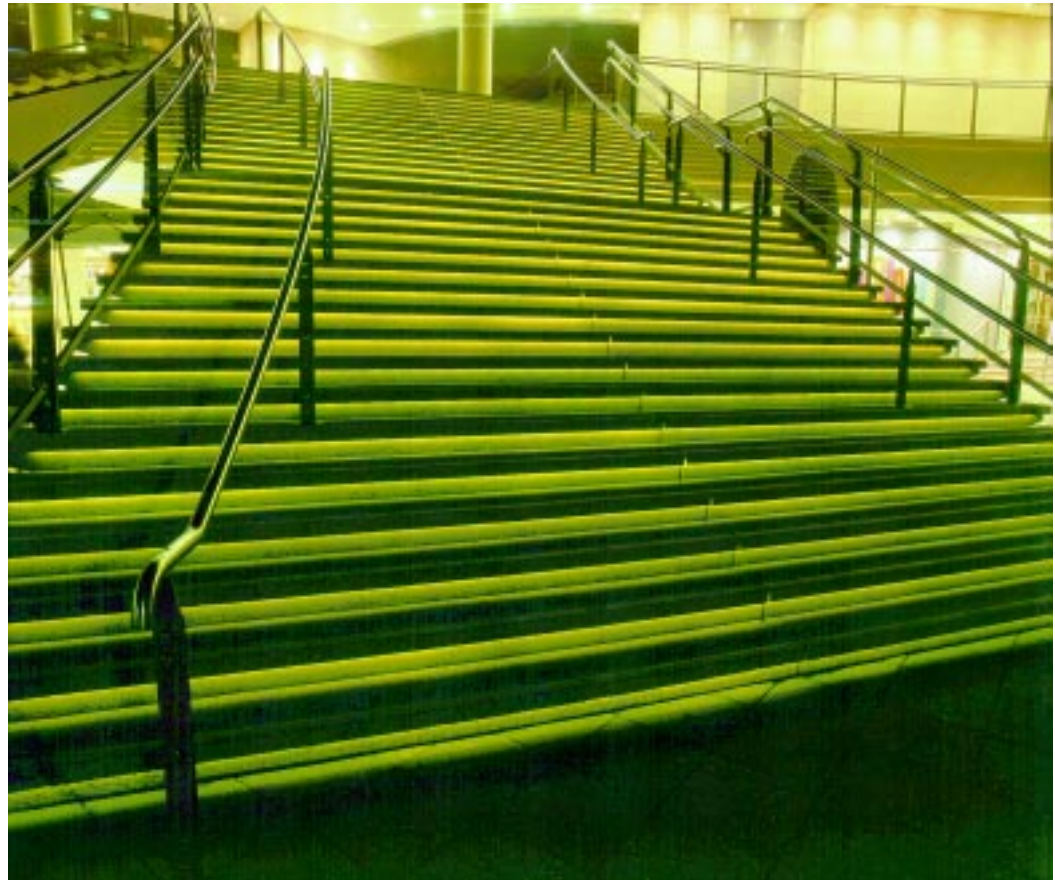
Upper level stair lighting
